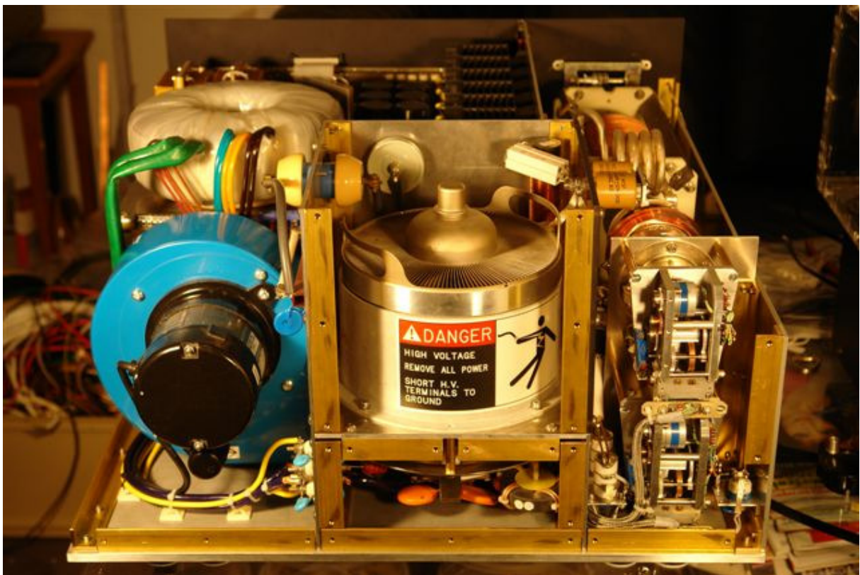
Fig. 10: Power amplifier without back board, the motors for the two vacuum capacitors on the right
